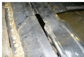
Old Draper Deck Front Joint (Spring Steel)
